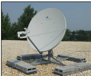
Figure 8: Typical Antenna with BUC and LNB
